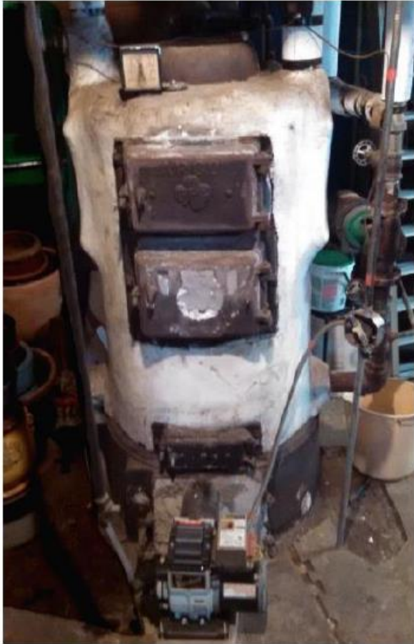
Boiler wrapped in asbestos insulation Picture from Expanded HEAT Loan Initiative Report , December 2015, E4theFuture.
